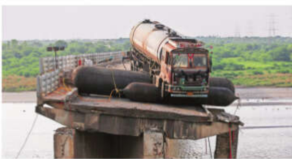
The tanker had been precariously perched on the bridge since July 9. Bhupendra Rana
